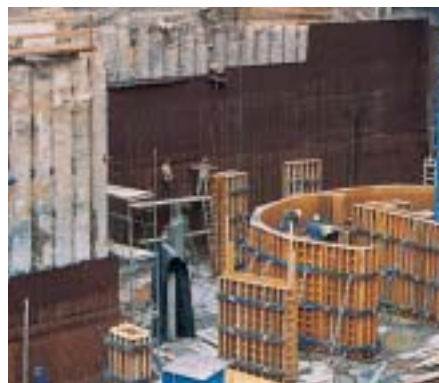
Underground garage of a Frankfurt hotel: Water emerging from the rocky subsoil is drained away by a DELTA®-MS seepage layer.
