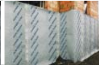
Permanent filtration and drainage.
