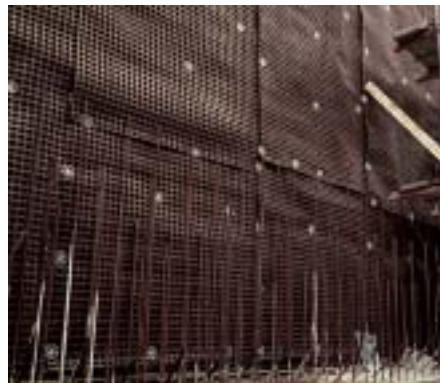
The Duisburg underground: DELTA®-MS 20 sheets installed between a reinforced curtain wall and the waterproof inner shell of the tunnel. This configuration permits structures to move without any unacceptable friction occurring between the curtain and the in-situ concrete wall.
