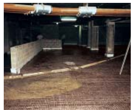
European Building, Brussels: The entire underground garage was put at risk by fluctuations in the groundwater level.
