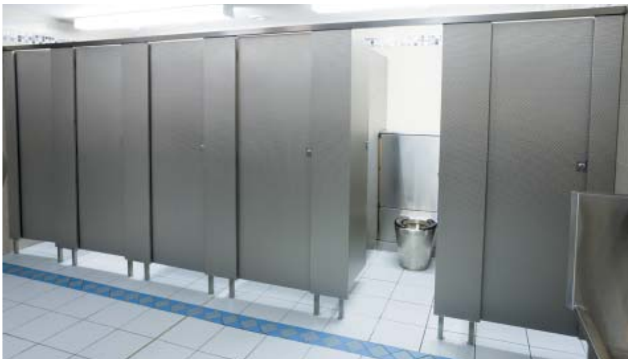
Stainless steel cladding to cubicles and cubicle doors. Olympic stainless steel anti-vandal WC pan.
