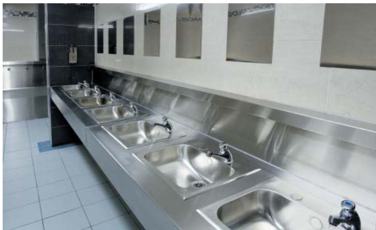
Stainless steel purpose made vanity sinks complete with stainless steel overshelf.
