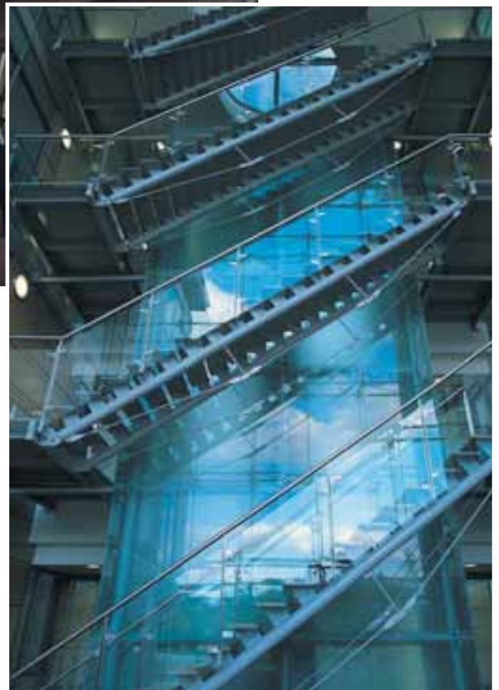
Four flight staircase complete with glass balustrading and timber treads and landings.
