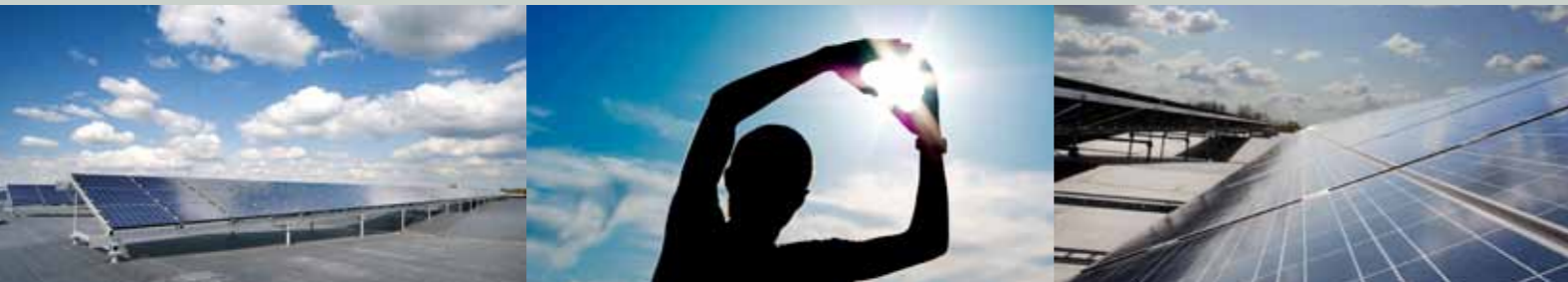
Reynaers - solar panels on roof of new distribution centre - Belgium
