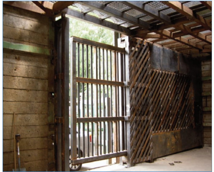
Automatic sliding gate to the new sleeping quarters
