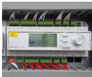
Controller box upgrade
