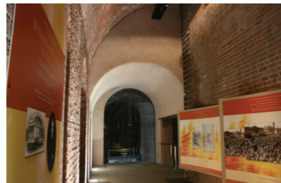
Newton damp proof membranes installed to the walls of St George's Hall, Liverpool, to fit the contours of the structure. The damp proof membrane acts as a permanent barrier and allows the damp walls to dry out
