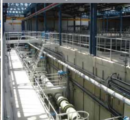
Headingly Water Treatment Works
