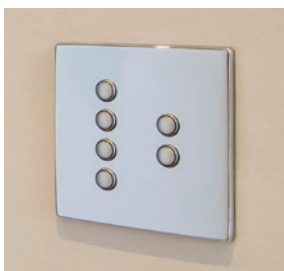
Mechanical button controllers in a Sheer CFX® plate design, finished in polished chrome were selected across the property to reinforce the minimalist and contemporary design theme.
