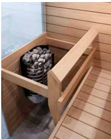
Ring Wall heater installed in the corner in Helo Deco Suvi interior.
