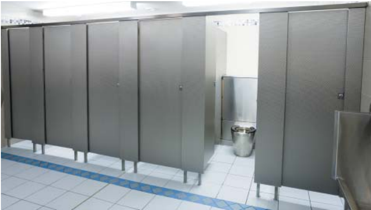
Stainless steel cladding to cubicles and cubicle doors. Olympic stainless steel anti-vandal WC pan.
