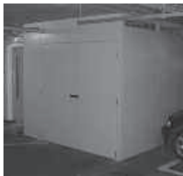
Here Sigma doors have been used as an access point to a secure enclosure.
