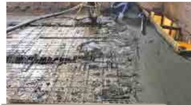
FORMATION OF THE COLLABORATING TOP CONCRETE SLAB ON THE EXTRADOS OF THE EXISTING SLAB USING LATERMIX BETON
