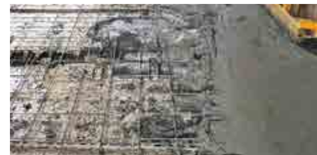
FORMATION OF A COLLABORATING CONCRETE TOP SLAB ON THE EXTRADOS OF THE EXISTING SLAB USING LATERMIX BETON
