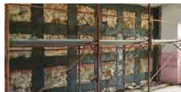
APPLICATION OF COMBINED AXIAL AND FLEXURAL FORCES AND SHEAR STRENGTHENING TO THE LOADBearing WALL
