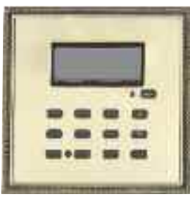
Air Conditioning Control
