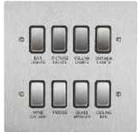
Bar Utility Switches
