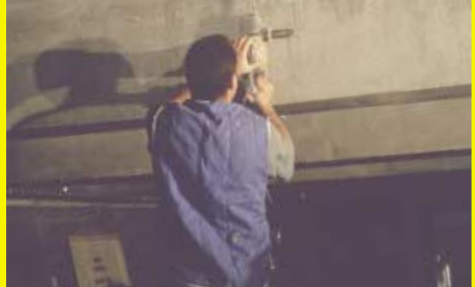
Surface preparation and sealing cracks prior to the shear strengthening of a slab in a building.
