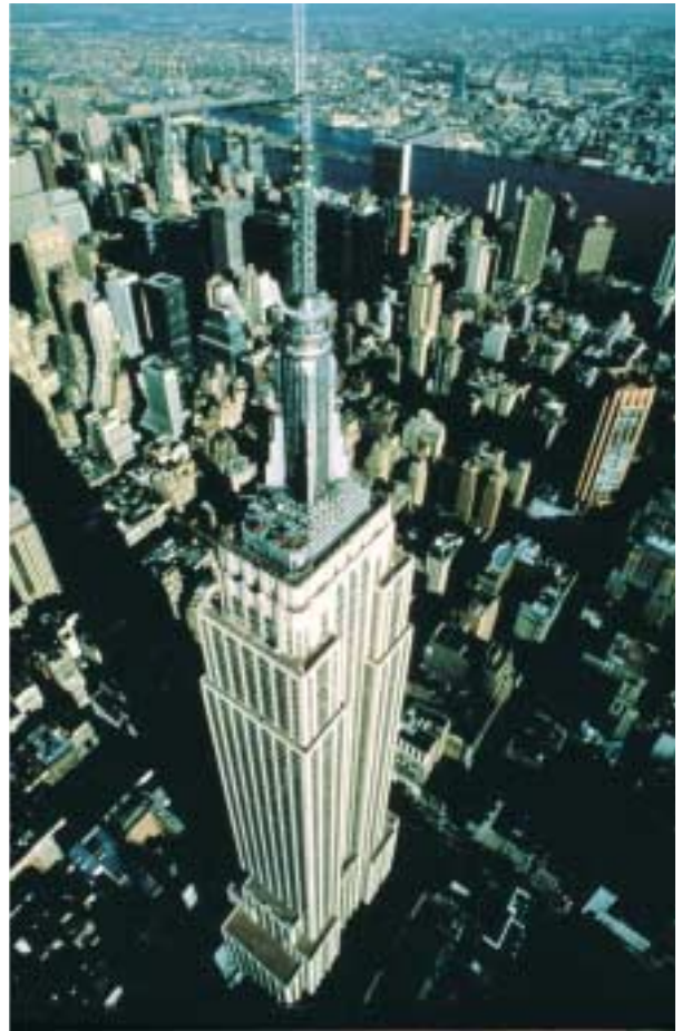
Sikaflex® sealants installed for long term re-sealing of all joints on the Empire State Building U.S.A
