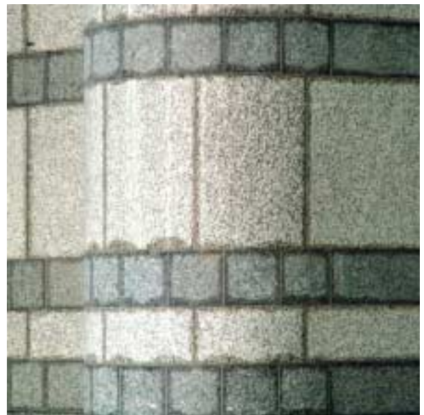
Typical polymer migration staining of marble panels - problem overcome using Sikaflex® polyurethane sealants
