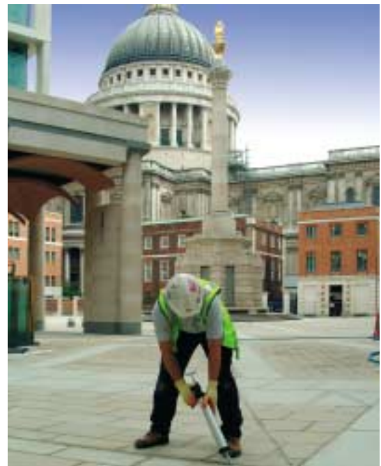
Specialist application of Sikaflex® Construction to sandstone paviour avoiding any future polymer staining
