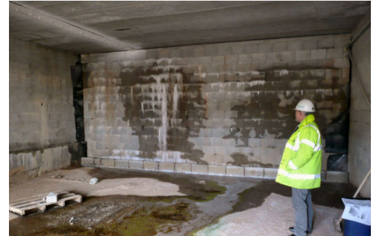
The property suffered from significant ground water ingress issues
