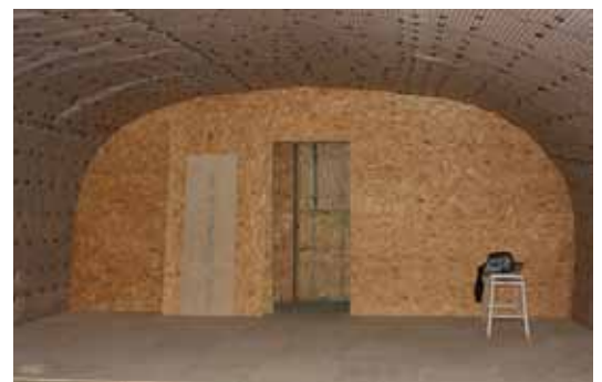
The tunnel is now fully protected from damp and is being transformed into a training facility
