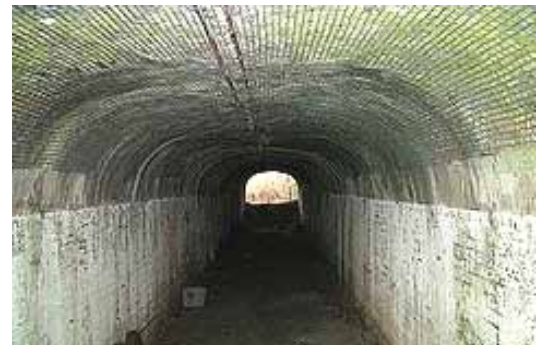
Charmouth Tunnel suffered from severe damp
