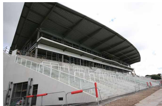
The new precast concrete grandstand at Ascot Racecourse required waterproofing to the construction joints
